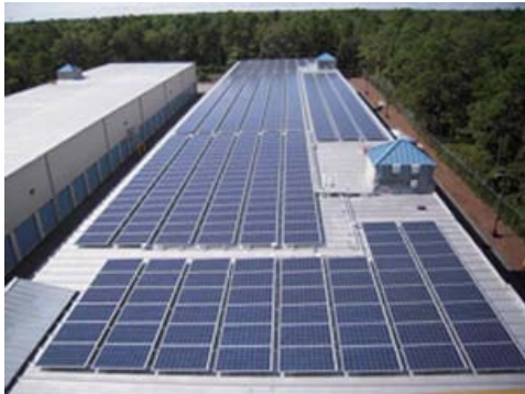
Solar Panel Array at Anchor and Flagship Self Storage facilities in Mashpee
